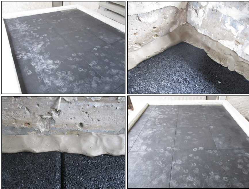
Images 5 to 12 Installation and sealing of the floor covering on the reference floor
